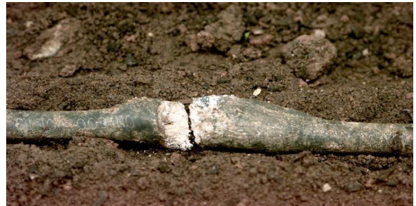
Figure 1: Corrosion Failure of Traditional 600 V Cable
