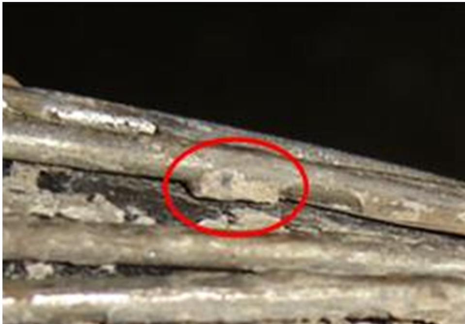
Figure 4: Metallic Shield Loss of Contact with Cable Insulation Shield Due to Mineralization
