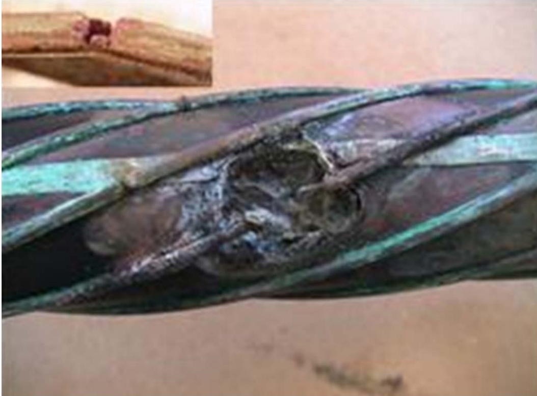
Figure 5: Exterior Arcing Due to Corrosion and Neutral Wire Break Causing Degradation to the Cable Core
