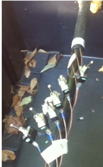
Figure 19: Cable System with Concentric Neutrals in Which Neutral Wires Can Be Switched In and Out Progressively
