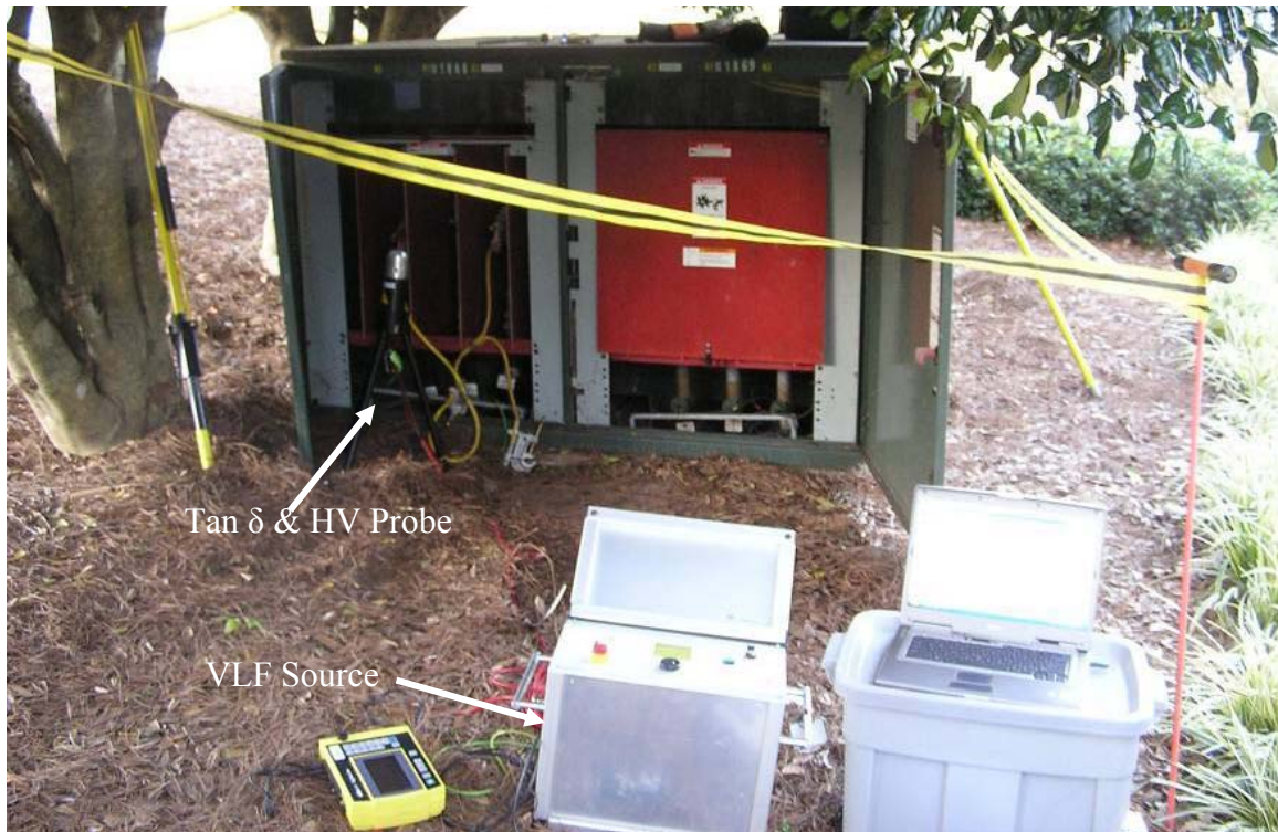
Figure 145: Tan \delta and Tan \delta Monitored Withstand Test Set Up
