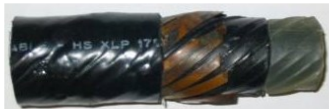
Figure 6: Cable Deformation Due to Elevated Temperature Operation
